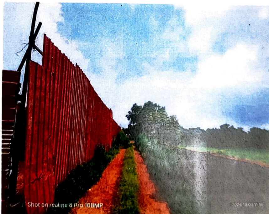
Plate 3: The road is separated from ongoing construction project by MS sheet fencing supported on MS Channels on the northern side and compound wall in the western side.
